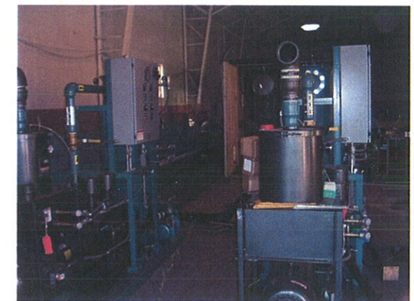
TWIN HVDPE SYSTEMS WITH SVE IN BACKGROUND
