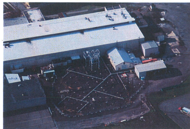
AERIAL PHOTO FOLLOWING SYSTEM INSTALLATION
