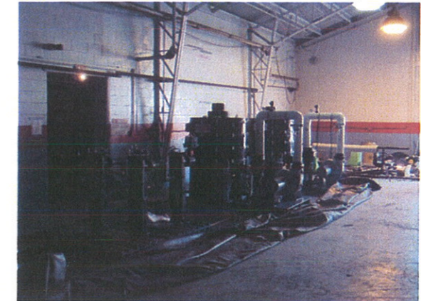
GROUND WATER TREATMENT SYSTEM DURING INSTALLATION
